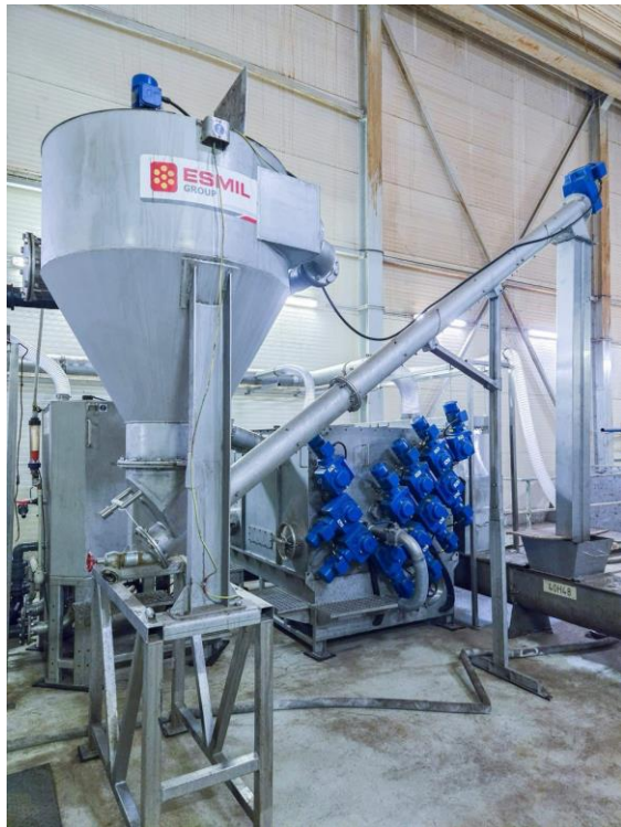
Figure 2 – Photo of the installation at the facility
